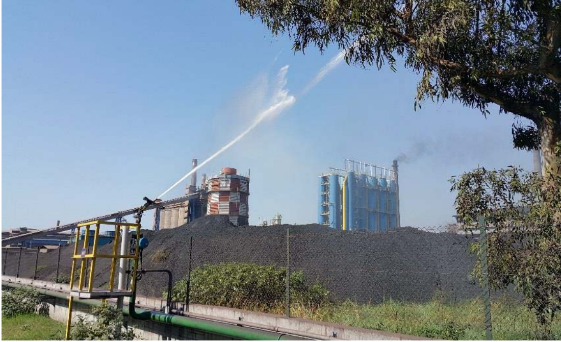
Installation of a Sprinkler System in the Coking Plant Coke Dust Storage Yard
