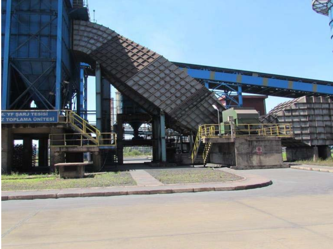
Installation of a Silobus Dust Evacuation System in the No. 4 Charger Dedusting System
